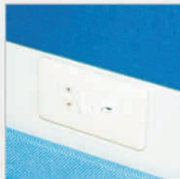
NETWORK, TELEPHONE & ELECTRIC SOCKETS
